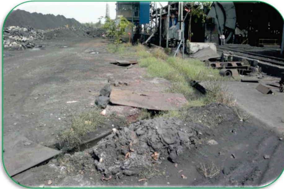
FIGURE 4.15 INADEQUATE WASTE WATER COLLECTION SYSTEM
