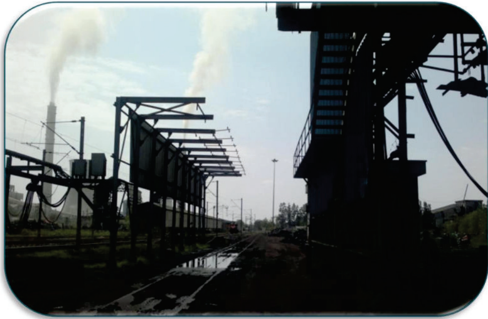
FIGURE 4.12 WATER SPRINKLING SYSTEM
