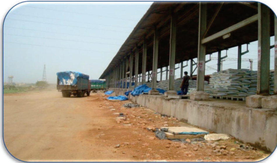
FIGURE 6.2 HAUL ROAD CONDITION AT FOOD GRAIN RAILWAY SIDING
