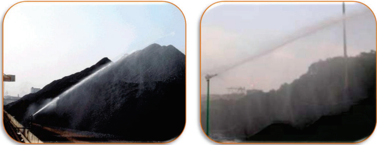
FIGURE 4.24 STOCKPILE WATER SPRINKLER SYSTEM
