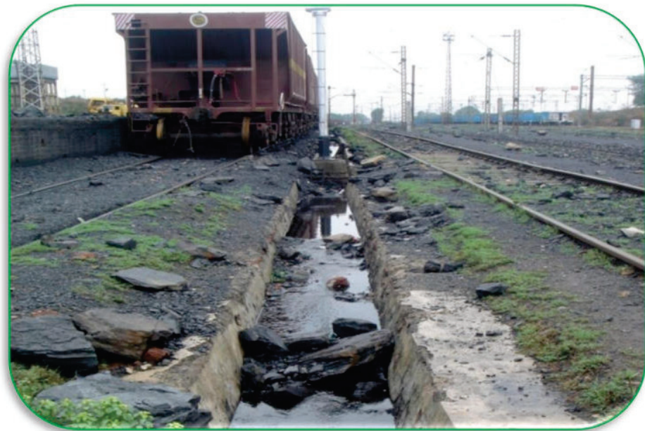
FIGURE 4.16 CHOKED CONDITION OF WASTE WATER COLLECTION SYSTEM
