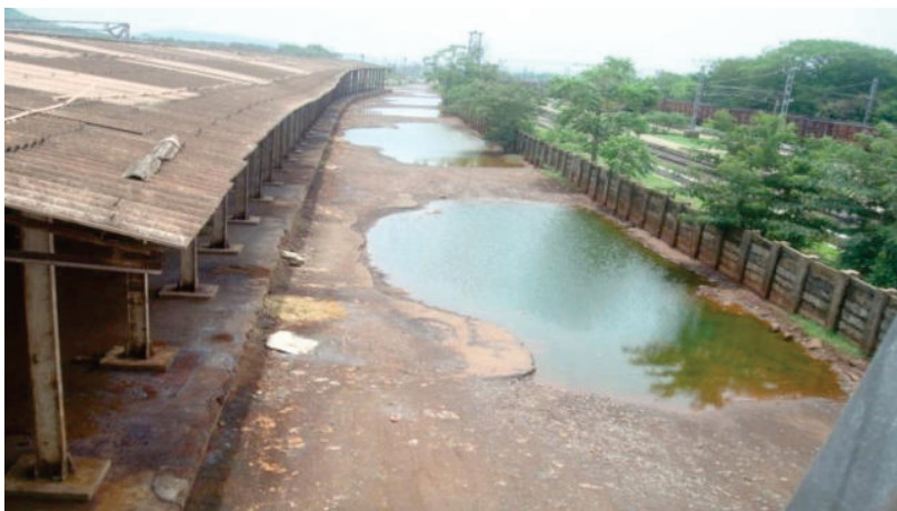
FIGURE 6.5 WATER LOGGING AREA AT SIDING
